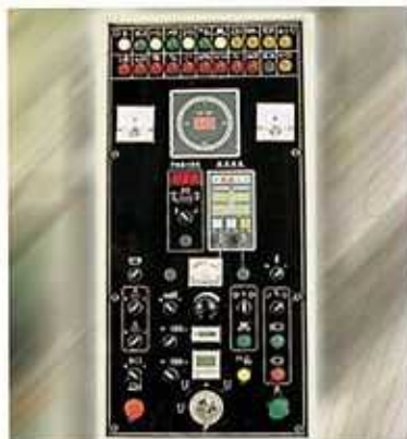
Operator Friendly Master Control Panel Display with signs, easy understanding and operation.
